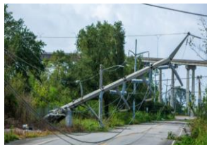
Hurricane Ida took out 9 of these high voltage powerlines into New Orleans.
