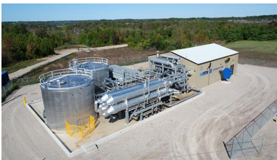
Portion of the Goderich A-CAES facility visible above ground
