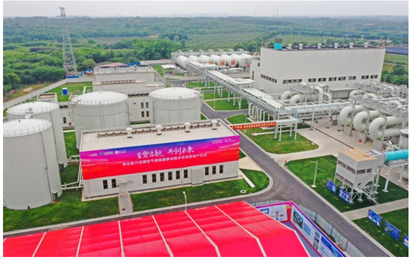
60 MW / 300 MWh salt-cavern CAES facility, located in the province of Jiangsu
