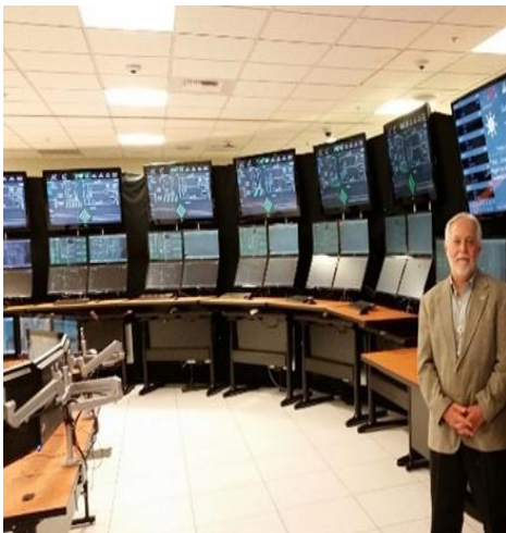
NuScale Control Room Simulator Photo Credit: Sid Crouch
