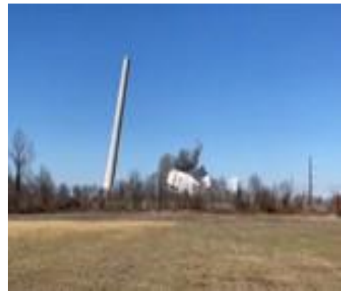
Logan Generating Plant Site Photo Credit: Starwood Energy
