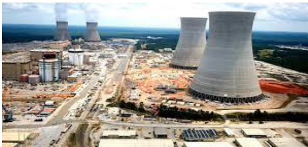
Unit 4 Hot Functional Testing at Plant Vogtle was announced completed on May 1. Photo Credit: Georgia Power Company
