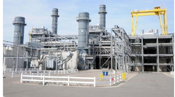
LV Sutton Plant (Gas replaced Coal) Photo Credit: Wilmington Star/News
