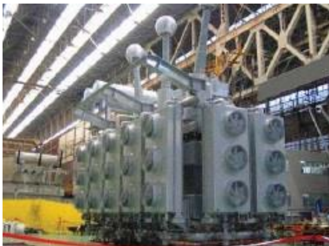
Hitachi Generator Step Up Transformer Photo Credit: Hitachi-tds.com
