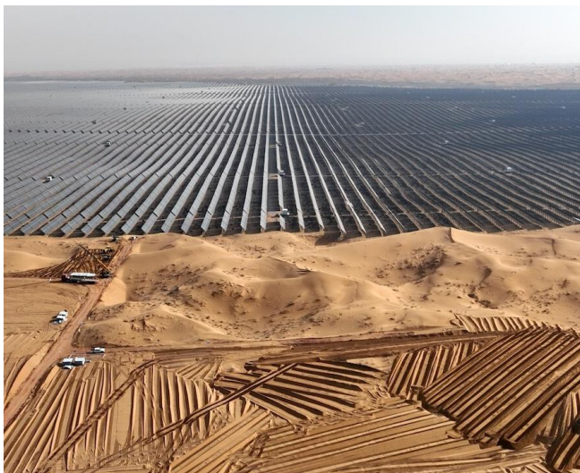
Solar Field Construction in China Image Credit: Yuan Hongyan / VCG via Getty Images
