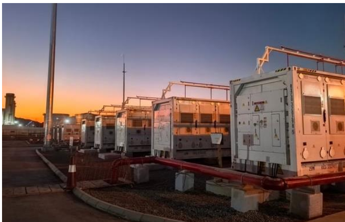
Bisha Project Battery Energy Storage Containers Photo Credit: PowerChina
