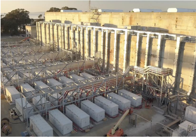
Vistra Energy's Moss Landing Battery Energy Storage Facility Photo Credit: vistracorp.com
